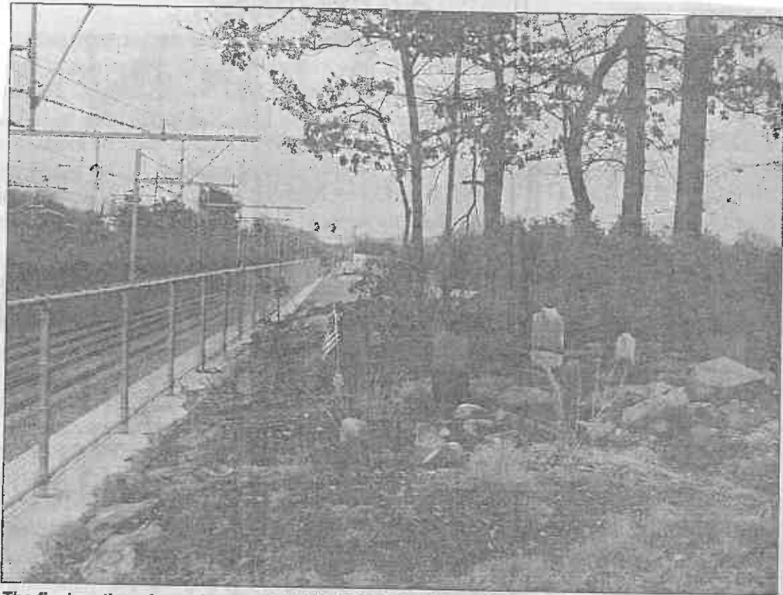
The final resting place of members of the Fones and Brown families lies beside the Amtrak train tracks in North Kingstown. Work crews recently erected a large, concrete retaining wall to protect the cemetery from erosion.
